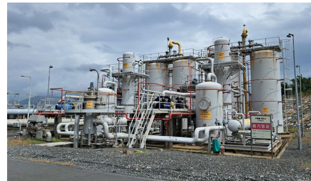
Yeosu Office Vapor Recovery Unit
